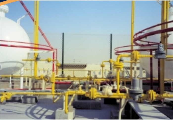
Example : hazardous area
